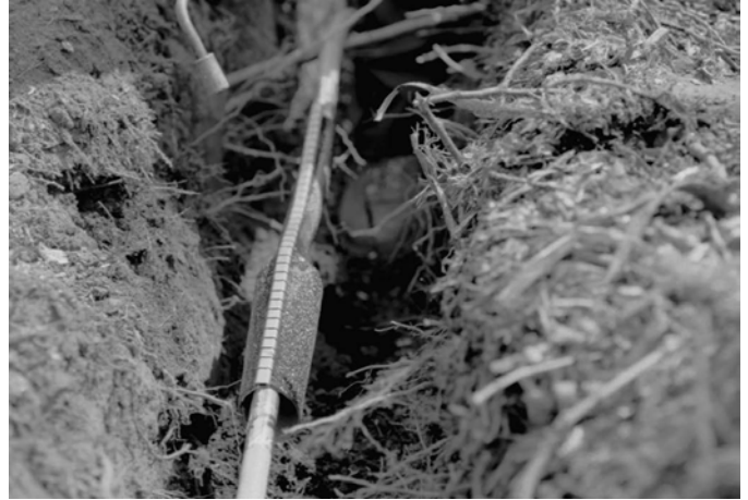
The CWST sleeve is simply wrapped around the damaged cable area and shrunk with a standard joiner's torch.
