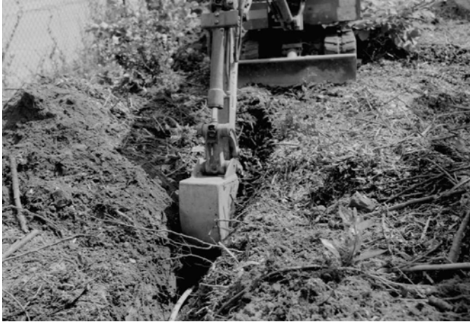
This cable jacket, damaged by an excavator, is quickly repaired.
